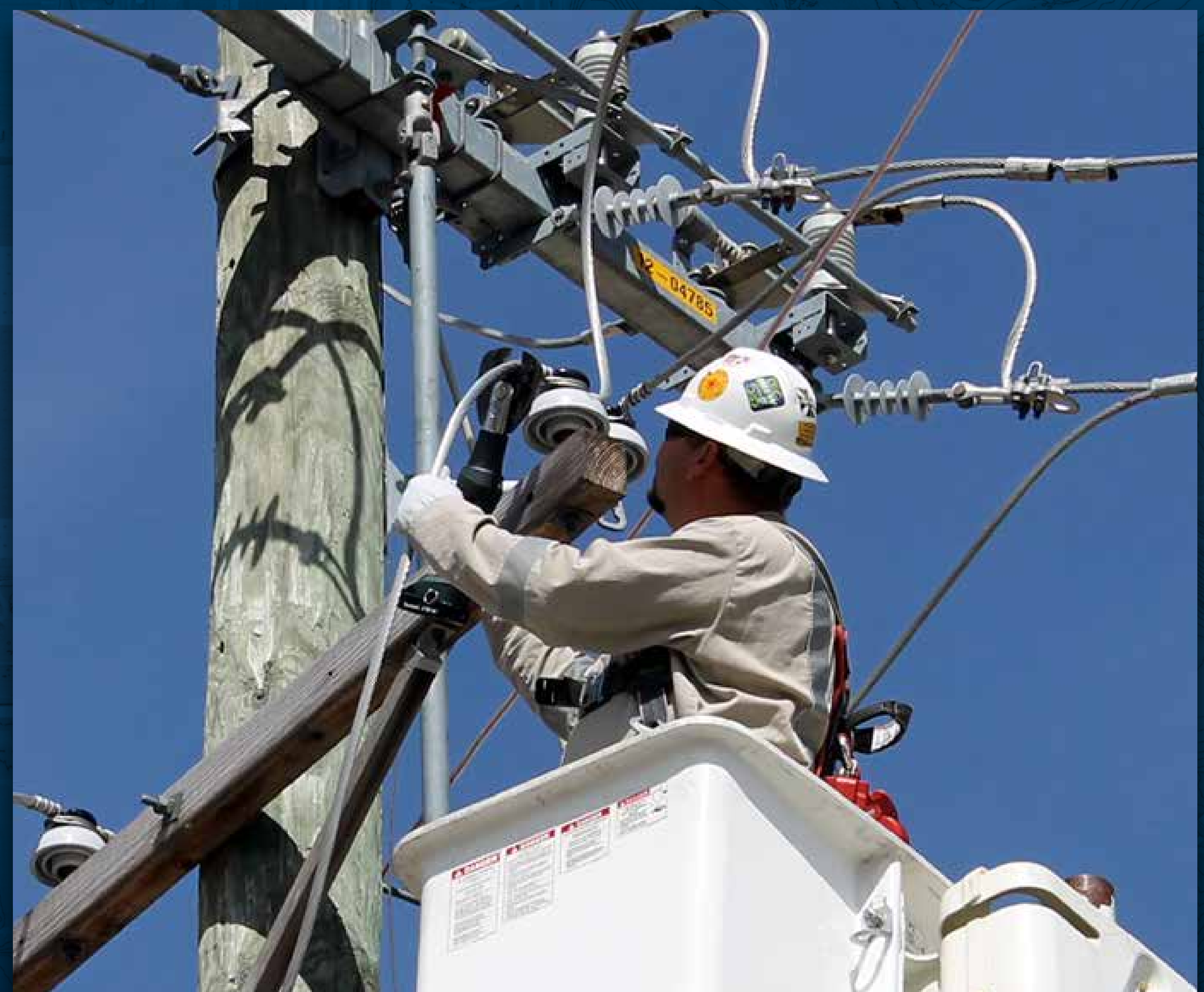
The final power source was removed Sept. 25, 2019
